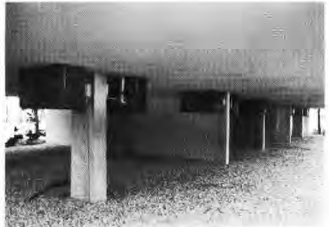
Figure 4.49. Elevated Condenser Units
