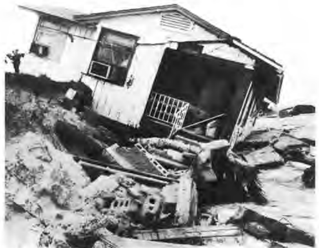
Figure 2.3. Erosion Caused This Foundation to Collapse.
